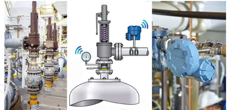
Figure 14: Rosemount 708 Wireless Acoustic Transmitters mount on piping adjacent to PRVs and steam traps to detect if they are functioning correctly or might be leaking. They are self-powered and send data via WirelessHART, so there is no need for any wiring.
